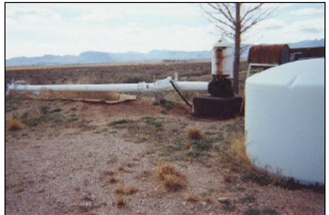
Irrigation well at headquarters
