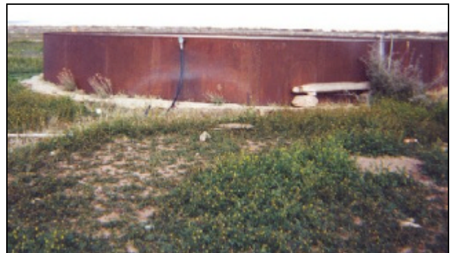
Borland pasture H 2 O storage and well which service pasture pipeline and drinkers
